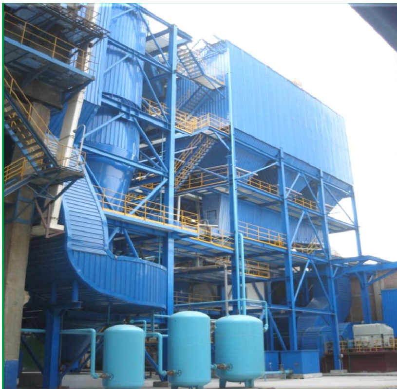
Figure 15 - SINOPEC Guangzhou Power Plant CFB System
