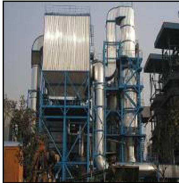
Figure 4 - JinJiang Demonstration Project
