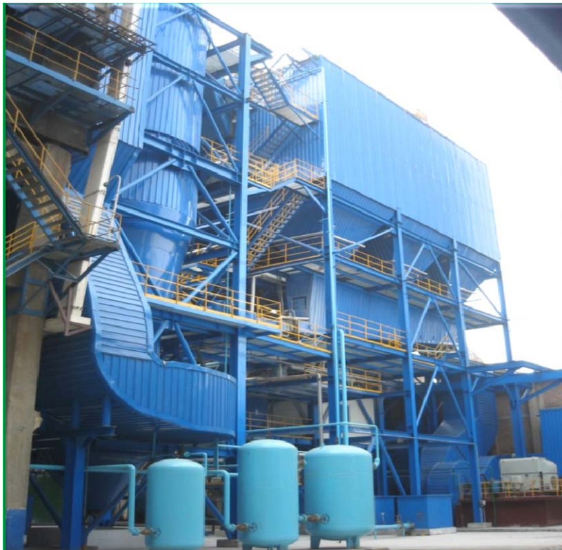
Figure 15 - SINOPEC Guangzhou Power Plant CFB System
